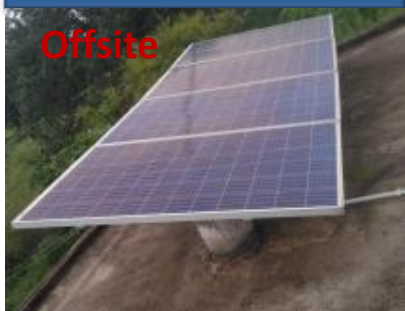
PV Solar Panel Installed at Intake Pump House
