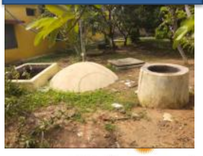
Kitchen food waste biogas plant
